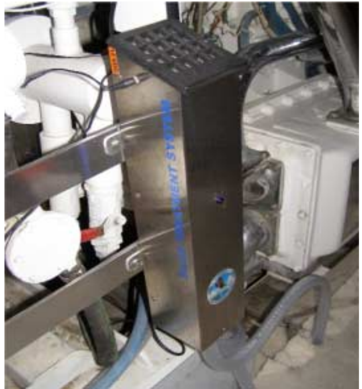
Holding Tank Ventilation System
