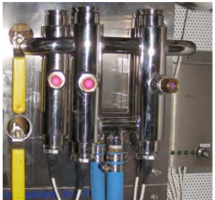
Advanced Oxidation Fuel Filtration System
